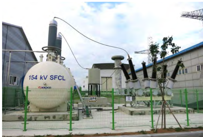
Figure 8. 154 kV SFCL developed by KEPCO. Photo courtesy of KEPCO.
