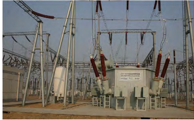
Figure 6. Innopower 220 kV/ 300MVA FCL. Photo courtesy of Innopower.
