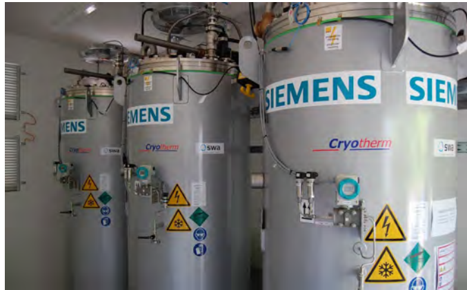
Figure 7. ASSiST FCL in Augsburg, Germany. Photo Courtesy of Siemens.
