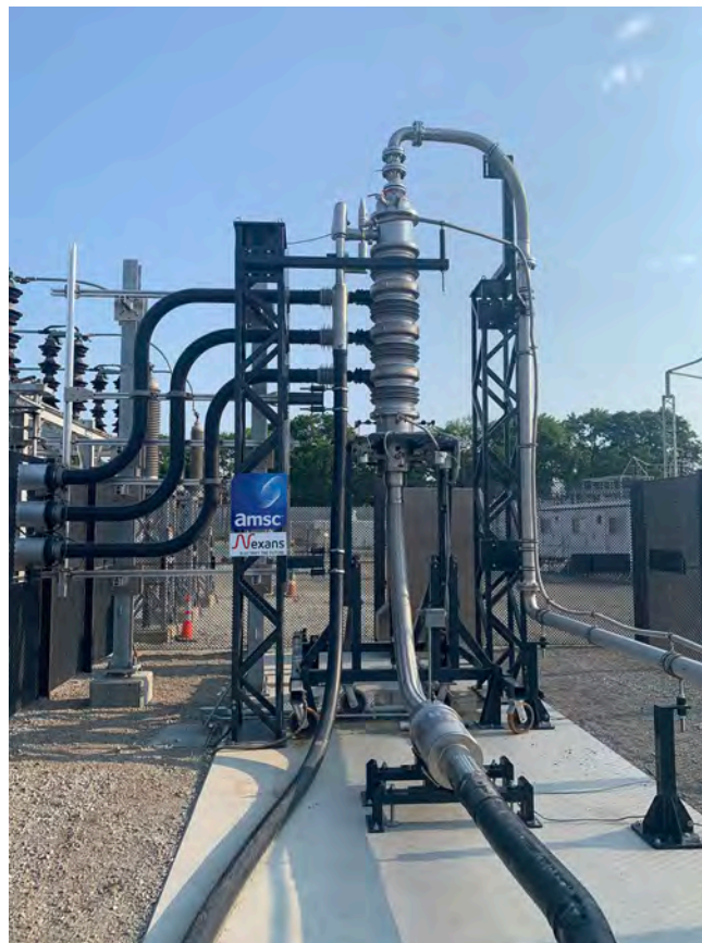
Figure 2. Termination of the Resilient Electric Grid cable in Chicago, Illinois. Photo courtesy of AMSC
