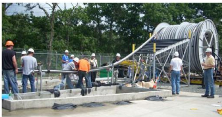
FIGURE 5. HTS CABLES CAN BE INSTALLED USING CONVENTIONAL CABLE PULLING TECHNIQUES. PHOTO COURTESY OF NEXANS.
